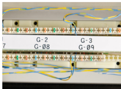
Terminal block labels
